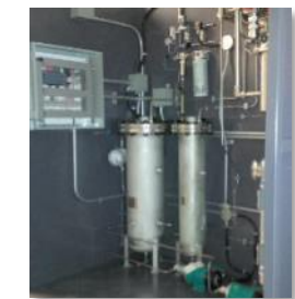
4. Oxygen and Feedwater Container
