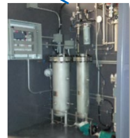
Oxygen and Feedwater Container
